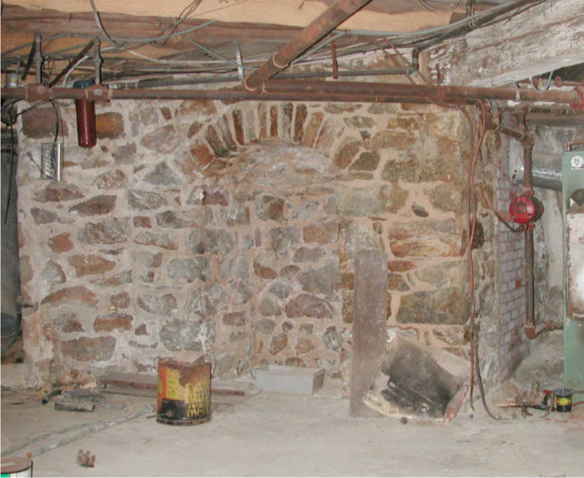
The relieving arch in the basement that supported the period II fireplaces and chimneys at the west end of the house.
