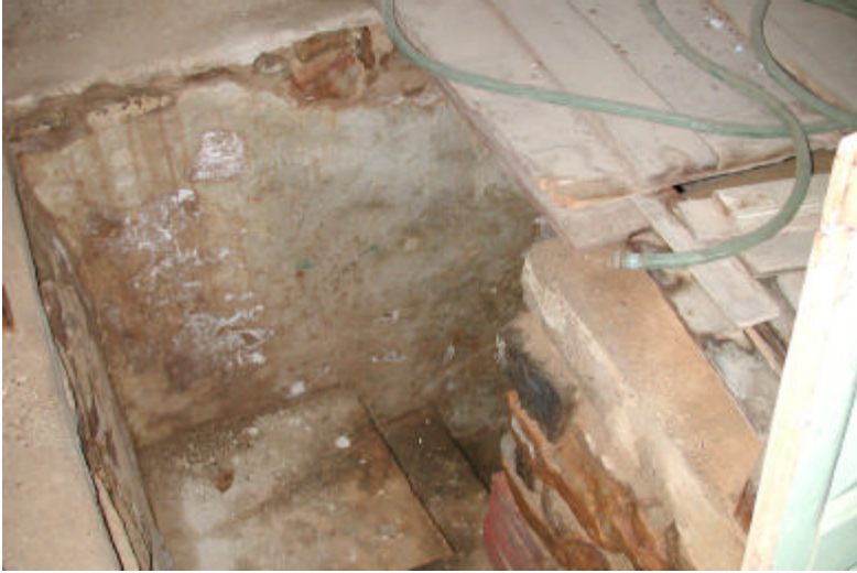
The view down the stairway leading from the cellar to the subcellar dairy.
